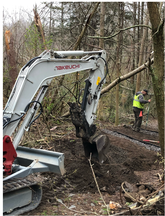
L.P. Murray and Sons make erosion control improvements to the Winnick Woods Trailhead
